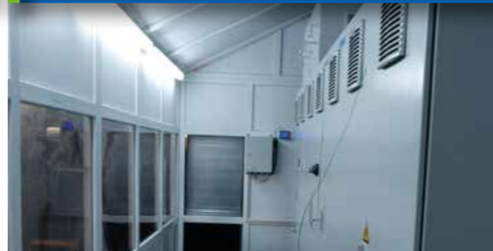
ELEKTRİK PANO ODASI / ELECTRIC CONTROL ROOM
