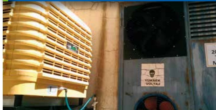
TRAFO ODASI / TRANSFORMER ROOM
