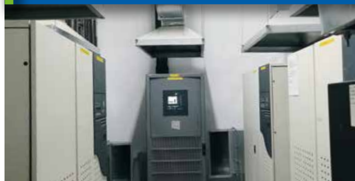
UPS ODASI / UPS ROOM
